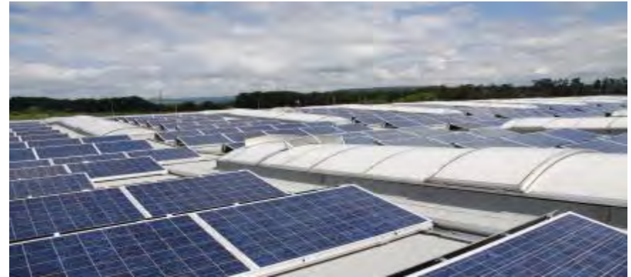
Schumacher Packaging, Forchheim; ca. 390 kWp
