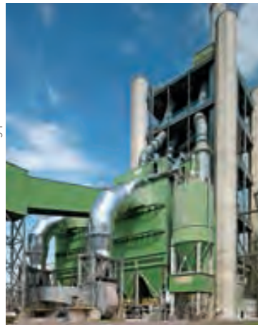
Dedusting plant for Cement Mill
